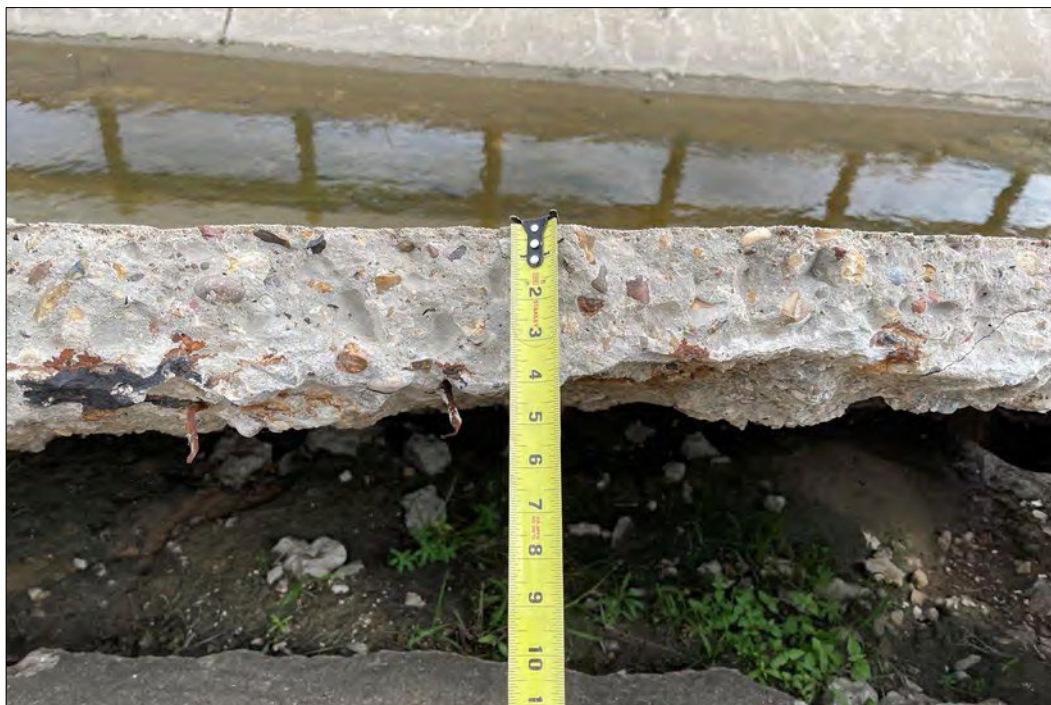
Photo 17: Displaced section of concrete slab that formed sloped sidewall of ditch
