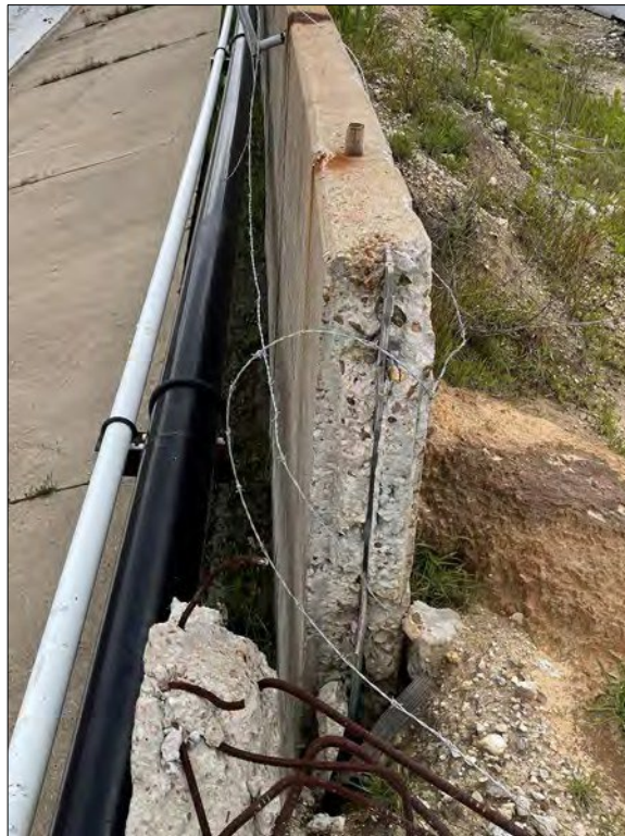
Photo 14: Torn waterstop and displaced wall. Upper section of wall that was displaced has been partially demolished during remediation efforts.
