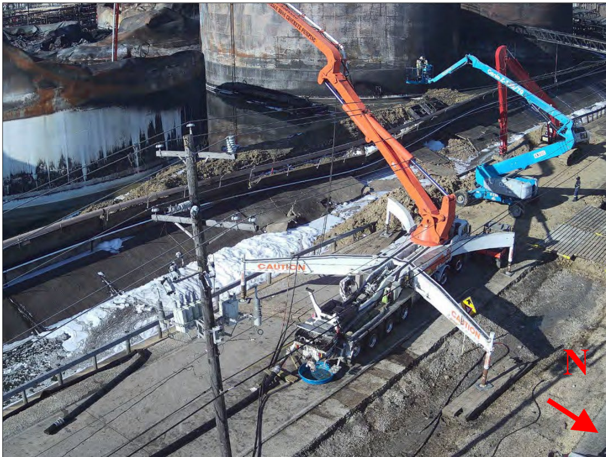
Photo 8: View of containment wall failure, after temporary dike wall was constructed 16
