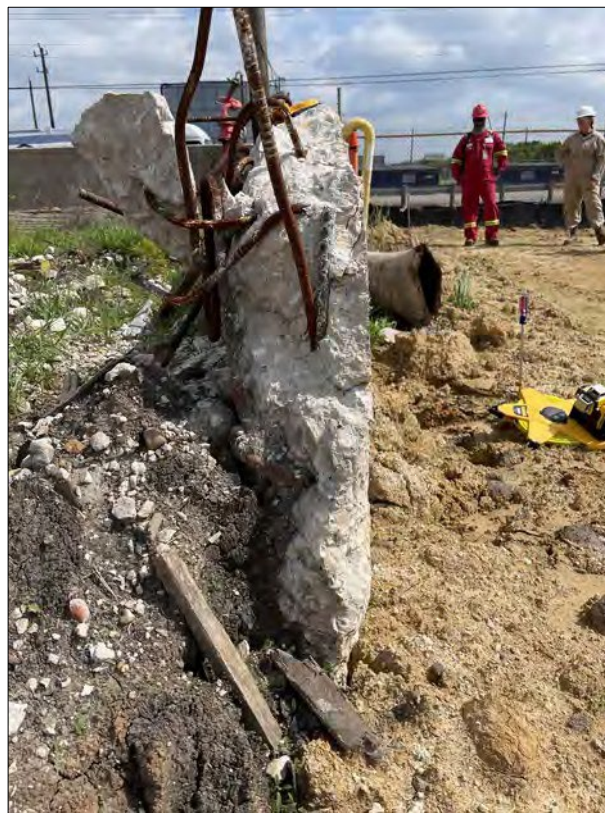
Photo 11: Exposed reinforcement at a section of the east containment wall where the wall was removed during remediation efforts
