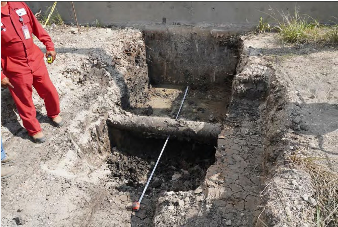
Photo 22: Containment wall footing excavation, south face of north wall, inside containment area
