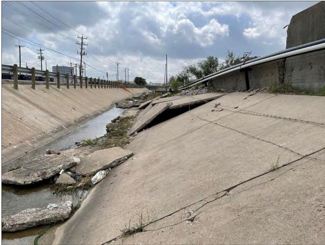
Photo 16: Damaged Section of Drainage Ditch, looking east
