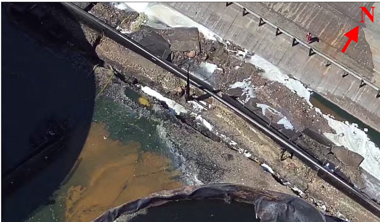
Photo 7: Aerial photo of containment wall failure after water flow stopped and before temporary dike wall was constructed 15
